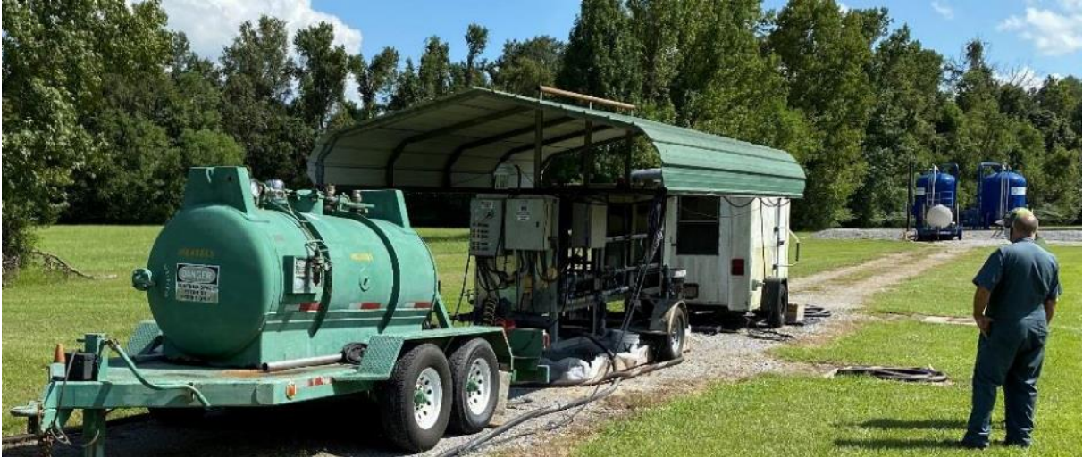
Scenic OU DTZ area showing molasses tank (green), injection well and carbon treatment unit (blue tanks in background)
