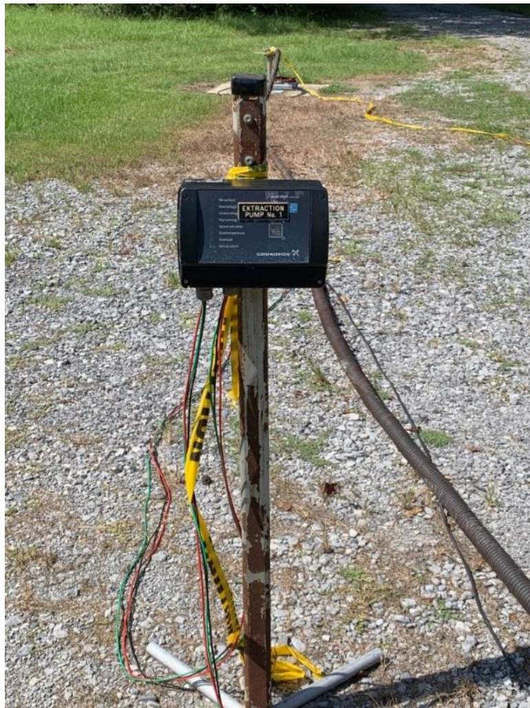
Extraction well at the DTZ of the Scenic OU
