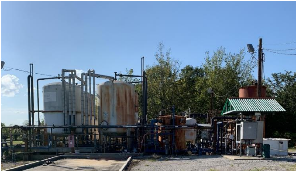
Stormwater treatment facility at the Brooklawn OU
