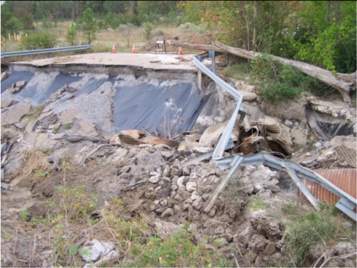
Photograph 27 – Bridge Failure, Scenic OU, Southwest 11/11/08
